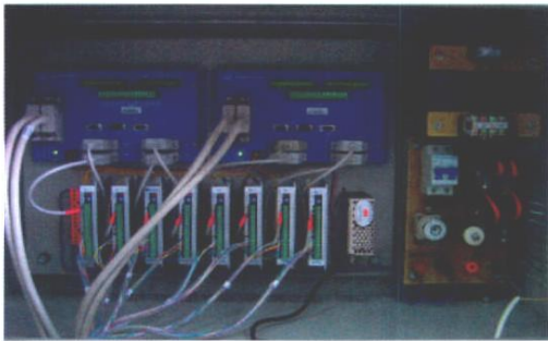
图4 电机控制柜内电子器件的线路搭接 Fig.4 Circuit connecting in the control cupboard
