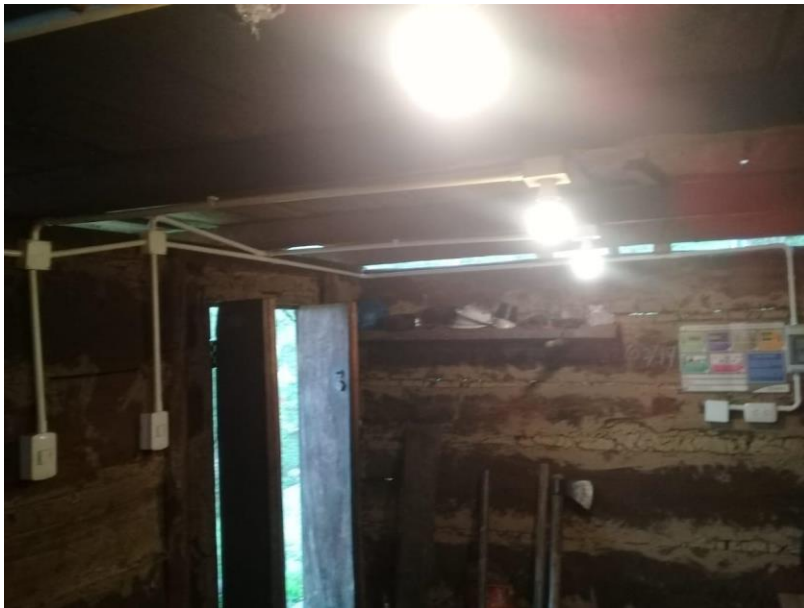
Figure 16 PV system equipment inside casa de campo
