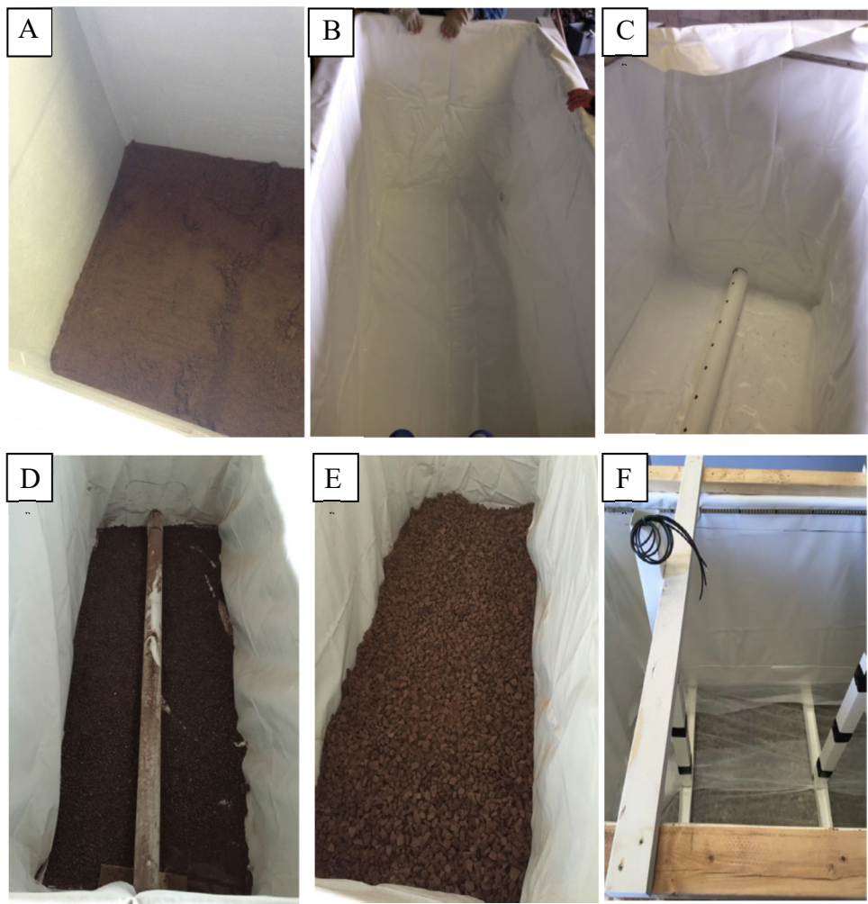
Figure 2-7. Boxes showing A) 1.5-2'' base sand layer, B) vinyl liner, C) drainage pipe, D) small gravel layer, E) 6A gravel to a level of ~2'' and, F) cross braces, sensor stacks, and filter fabric on bottom.
