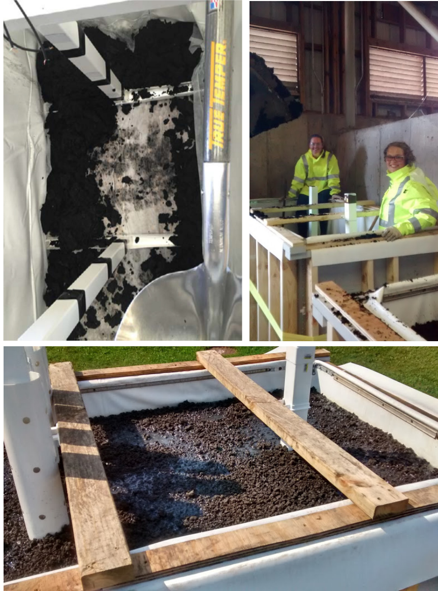
Figure 2-8. Final construction of pilot scale boxes. A front-end loader was used to evenly fill boxes with biosolids.
