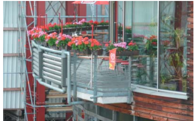
Solar thermal is also used extensively Here on the balcony of the cycle hub
