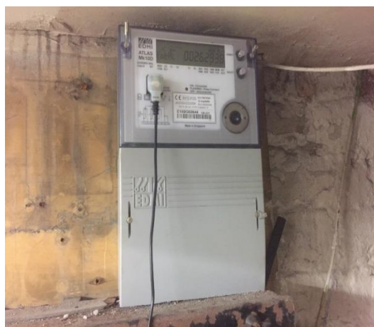
Figure 19 Main incoming electricity meter monitored with an optical metering device.
