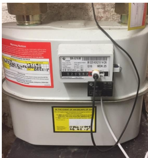
Figure 18 Gas meter reading equipment
