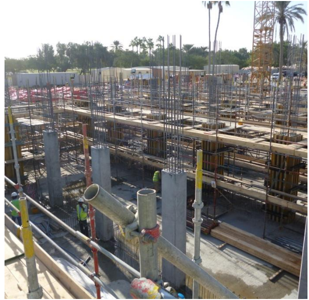
Fig.7. Construction site image shows static occlusions (i.e. scaffolding) due to daily construction activities
