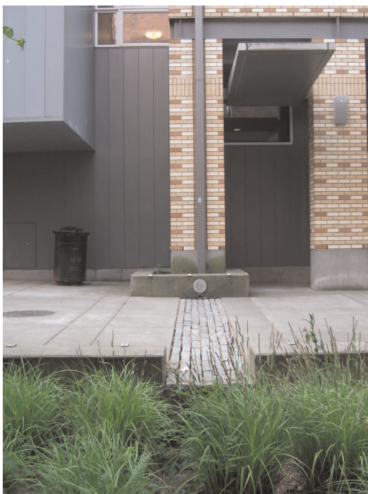
Figure 2. Downspout issuing into rain garden, Portland, Oregon
