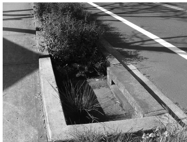
Figure 8. Bioswale inlets in the USA
