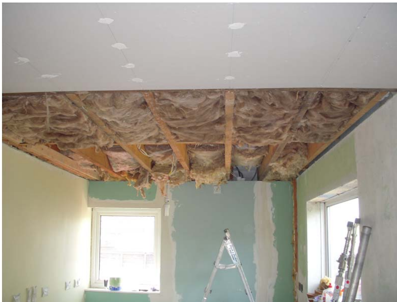
Case006 participant photo of work progression – process of insulating the ceiling/upper floor
