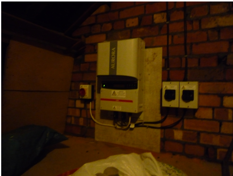
Case0005 photovoltaic inverter
