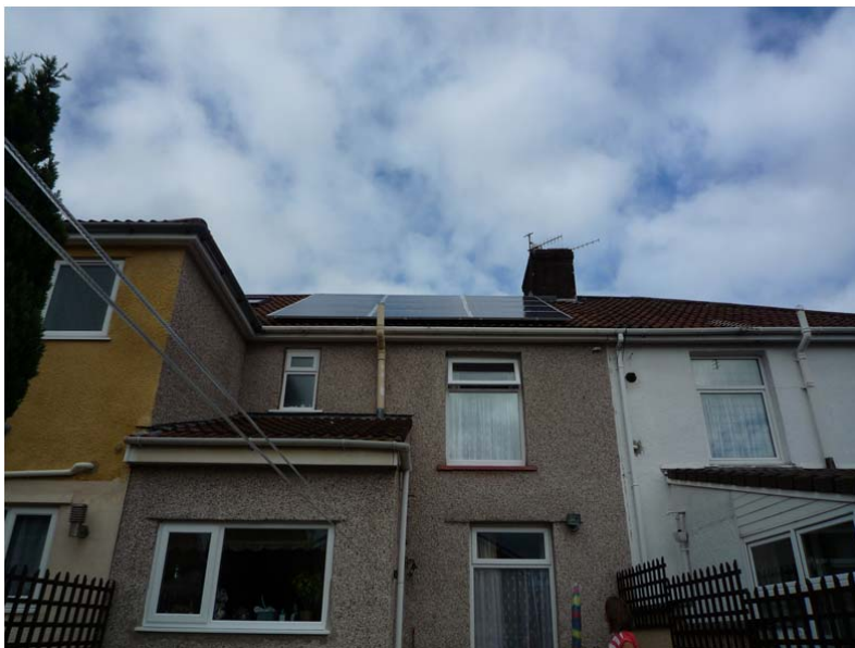
Case022rear elevation including photovoltaic panels
