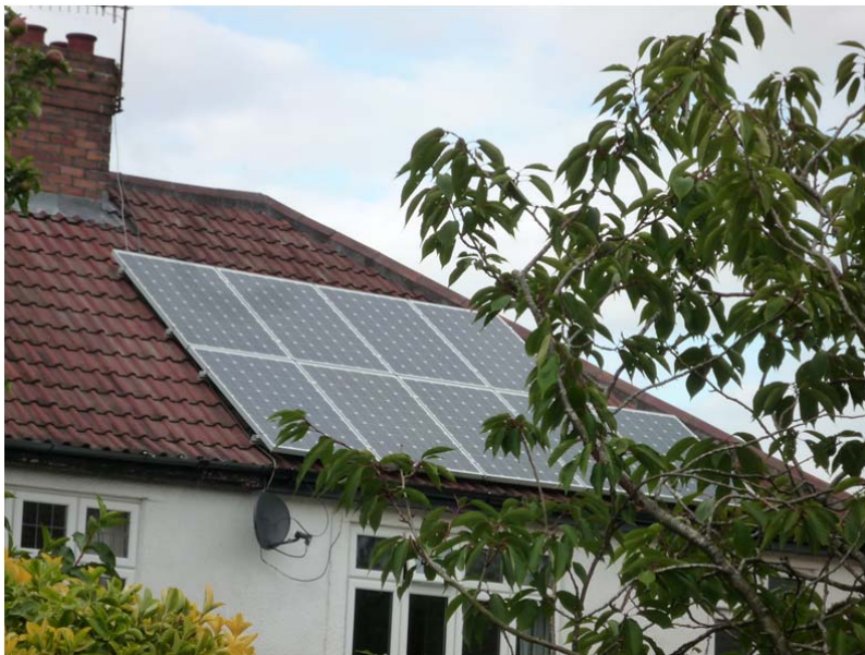
Case004 photovoltaic panels to the rear of the property
