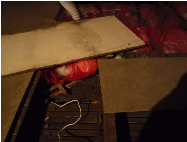
Case004 lack of loft insulation
