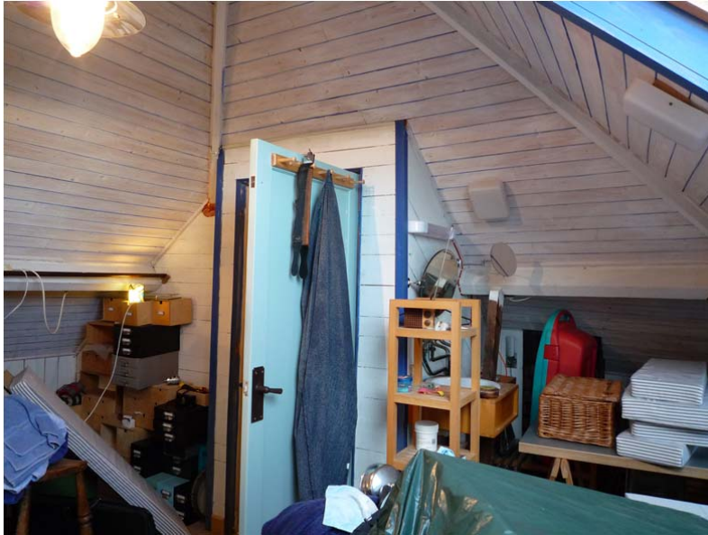
Case025 loft space ('do-it-yourself' conversion without Building Regulations)
