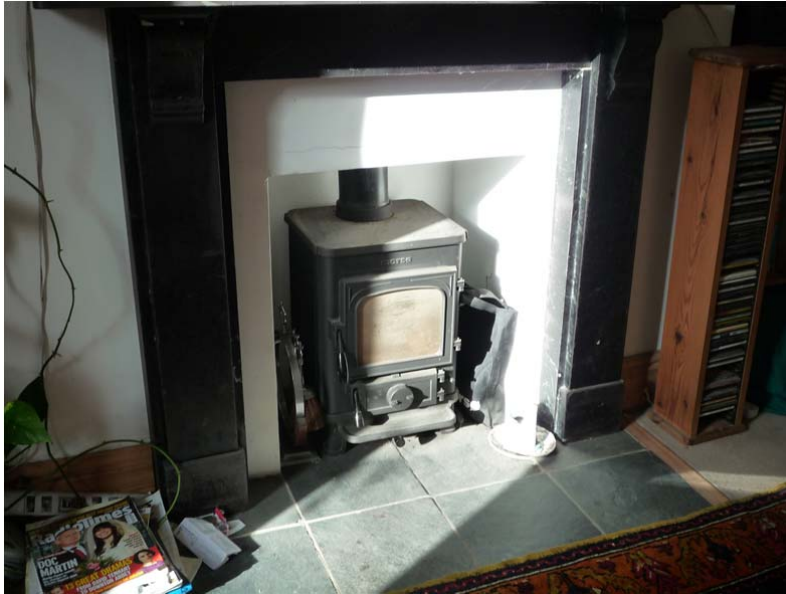
Case017 wood burning stove (lounge)
