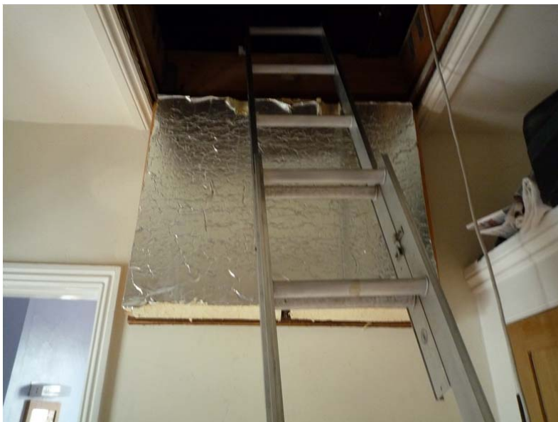
Case021 insulated loft hatch
