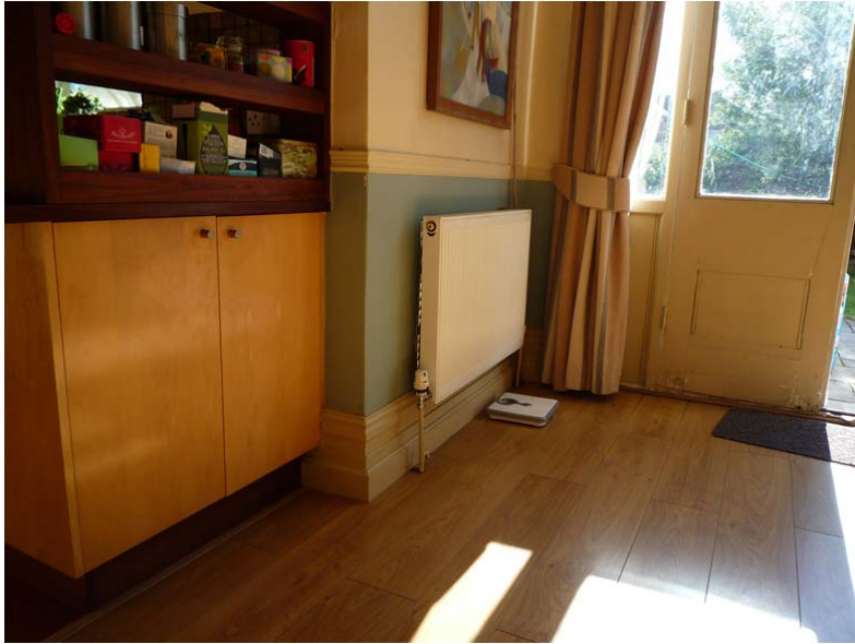
Case015 kitchen-dining area showing finishes, double panel radiator and single glazed timber French door leading to garden
