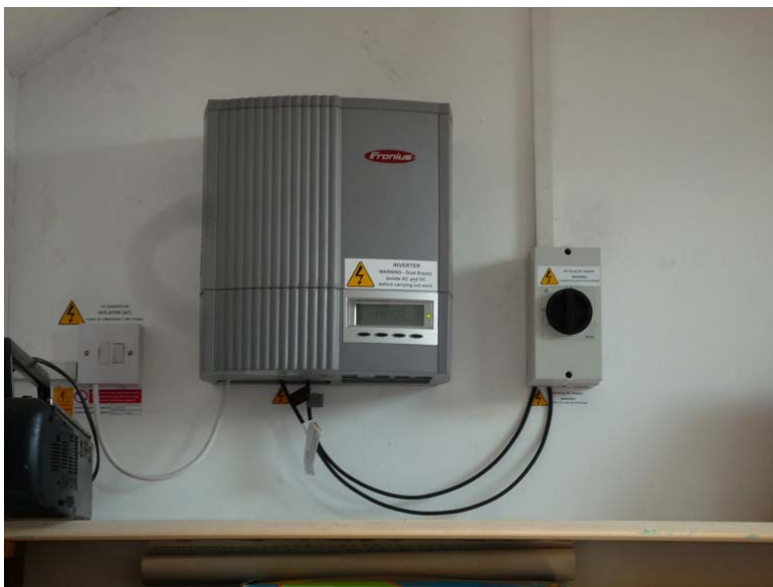
Case009 photovoltaic inverter
