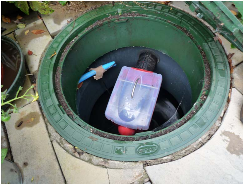
Case021 rainwater recycling system
