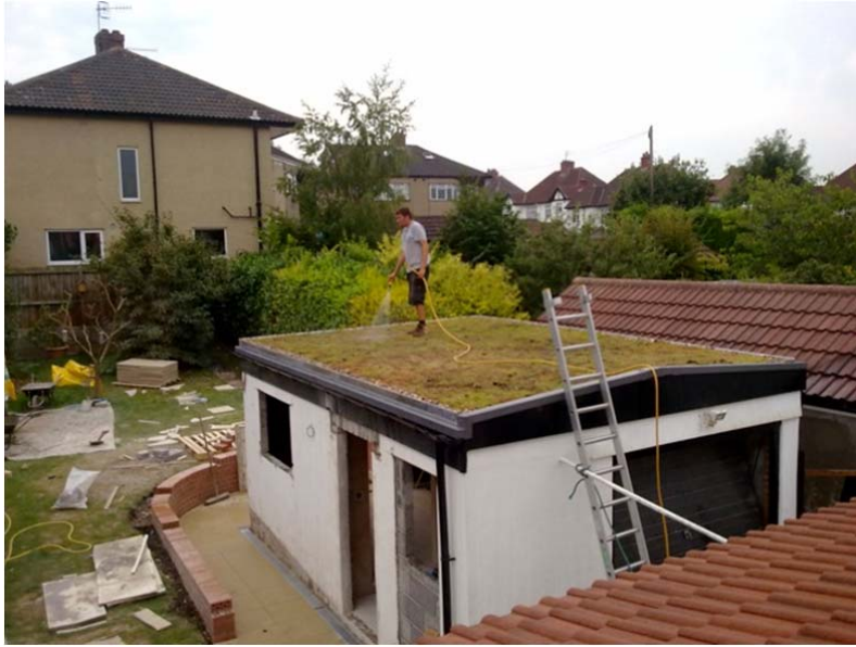
Case007 fully installed green roof
