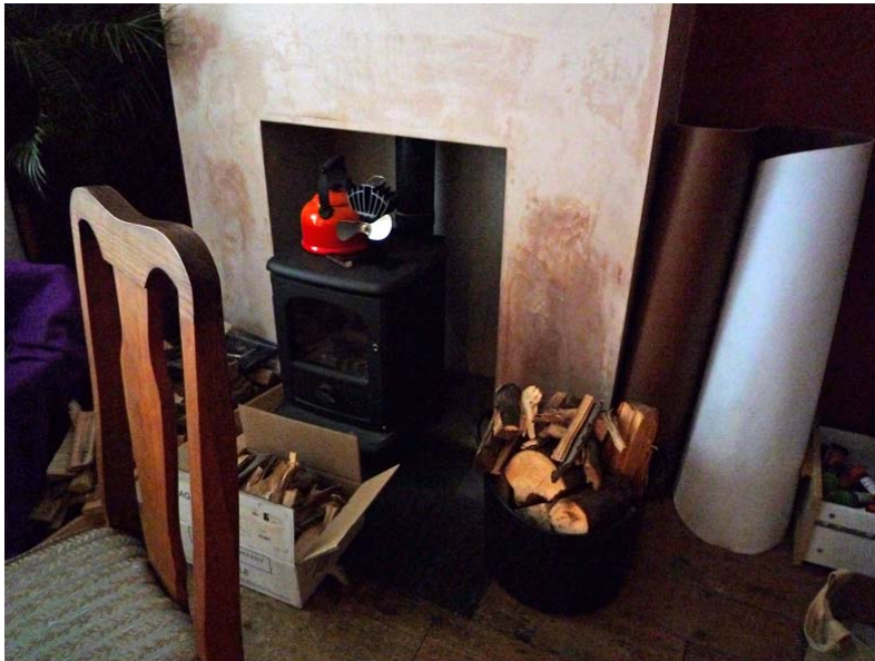
Case002 woodburning stove (kitchen-dining area)
