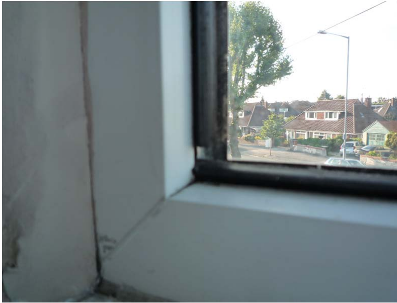
Case014 double glazing - deterioration
