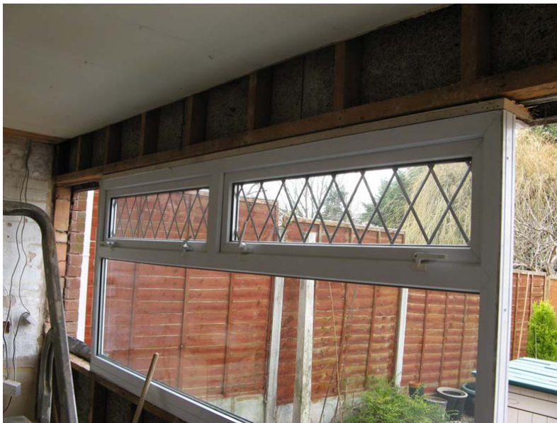
Case013 participant photograph of cross wall - timber frame with 'stramit' exposed during refurbishment
