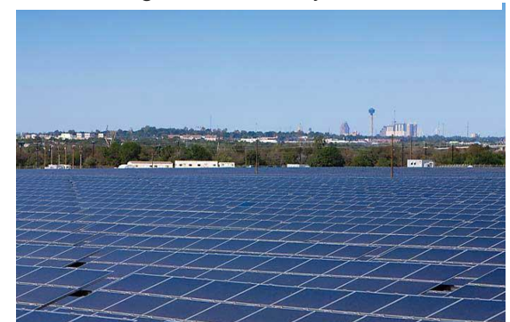
Blue Wing Solar PV Array ,San Antonio
