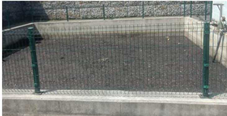
Figure 1: Leachate storage tank.
