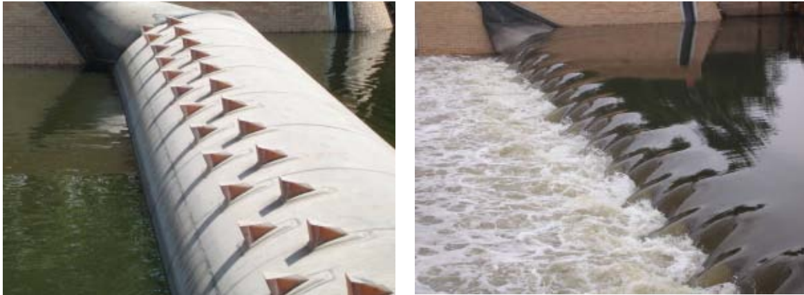
Figure 12: Weir Bahnitz east of Berlin: row of breakers (left), weir in operation (right)
