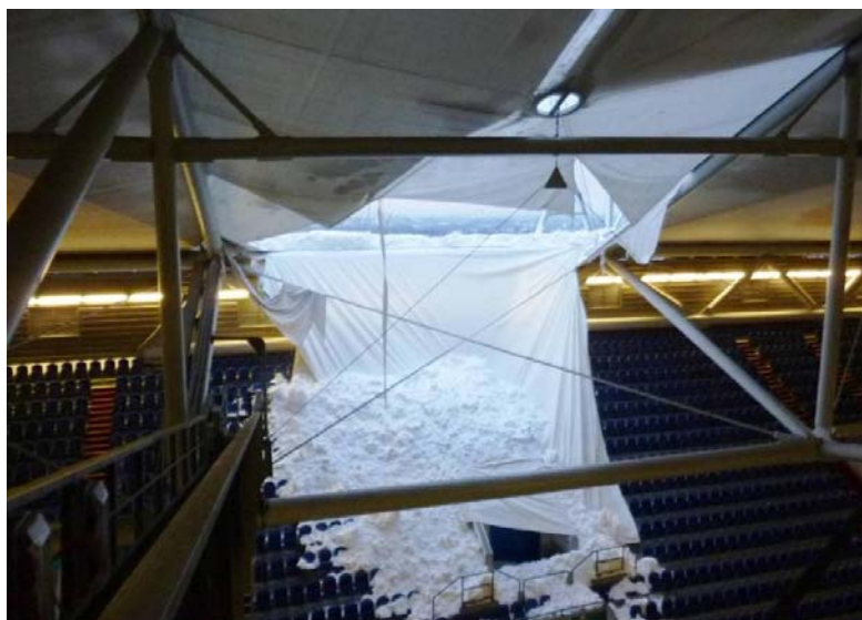
Figure 22 Veltins-Arena, snow loads on the stand after failure of a roof panel
