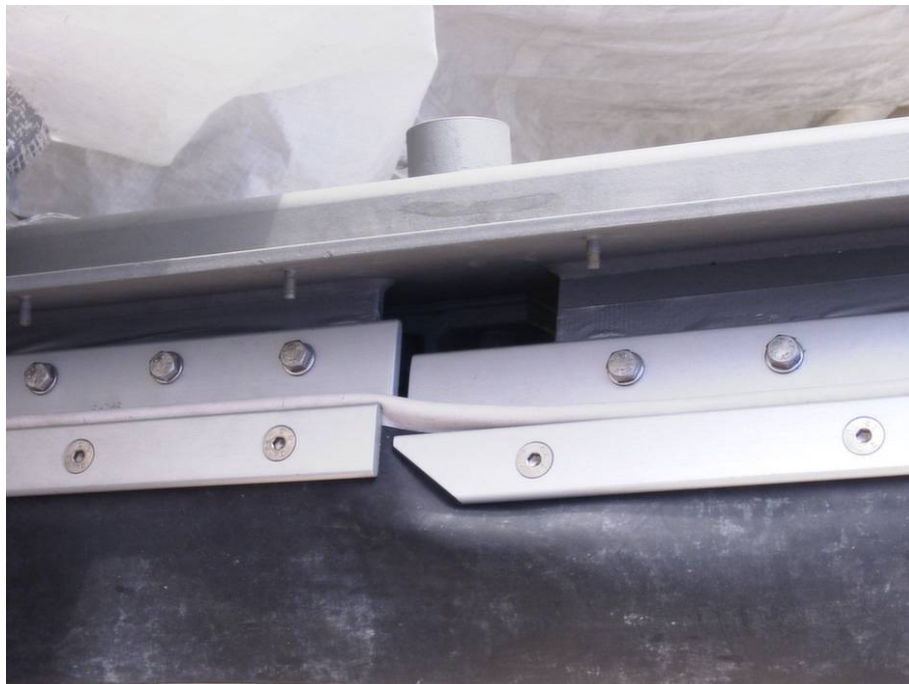
Figure 20 Offset of clamping plates fixed to steel structure
