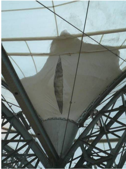
Figure 25 Main station Dresden, ruptured funnel with snow filling
