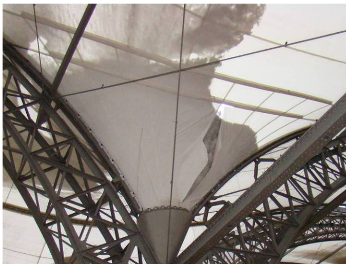
Figure 26 Main station Dresden, ruptured funnel with snow filling
