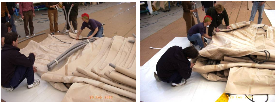
Bild 4 Folding of excess area at a large membrane panel, mind the foam rolls at photo on left, these are too small and do not prevent kinks when fabric is folded
