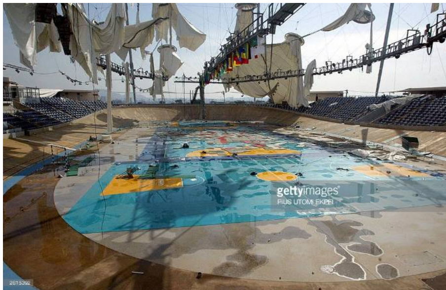
Figure 31 Velodrome Abuja, Membrane damaged after thunder storm © Getty Images
