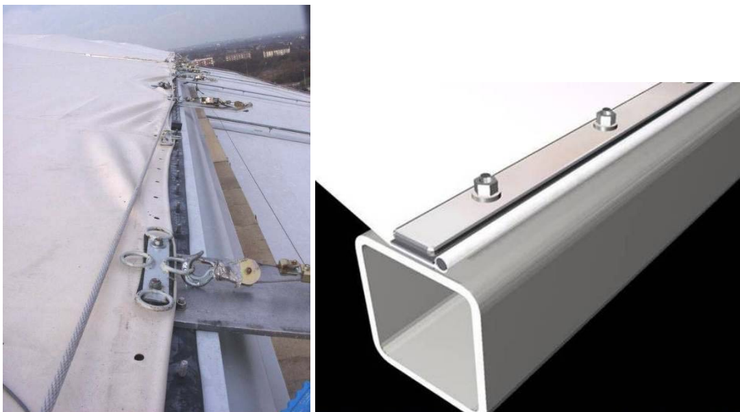
Figure 16 Clamping edge, planned details on RHS, LHS shows situation during installation with auxiliary clamps
