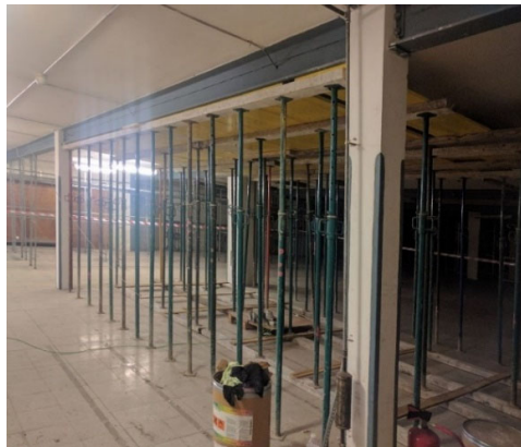
Figure 8. General view of the shoring and formwork on basement level -2 for safety reasons.
