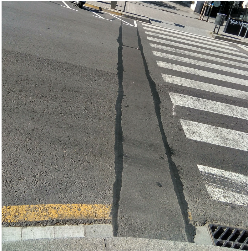
Figure 26: When a new infrastructure is disposed through the streets of a city, in most cases the only option is to remove the asphalt and dig, therefore disrupting traffic while the infrastructure is being disposed. OWN ELABORATION.
