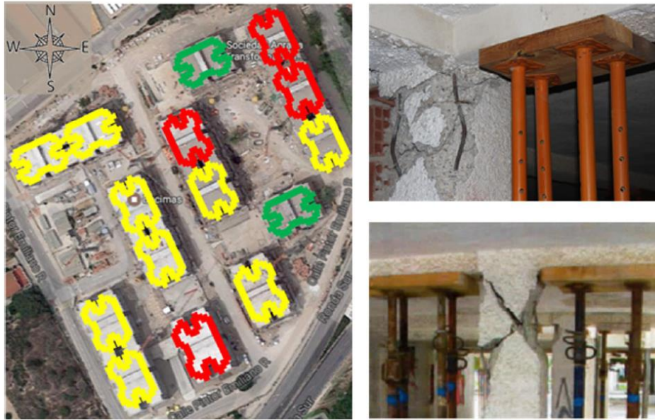
Figure 5. Plan view of the buildings located in San Fernando neighbourhood affected by the Lorca earthquake. Green colour indicates that the building was not damaged; yellow colour means that the damage is repairable and red colour indicates that the building is holding extensive damage and that there is risk of collapse.
