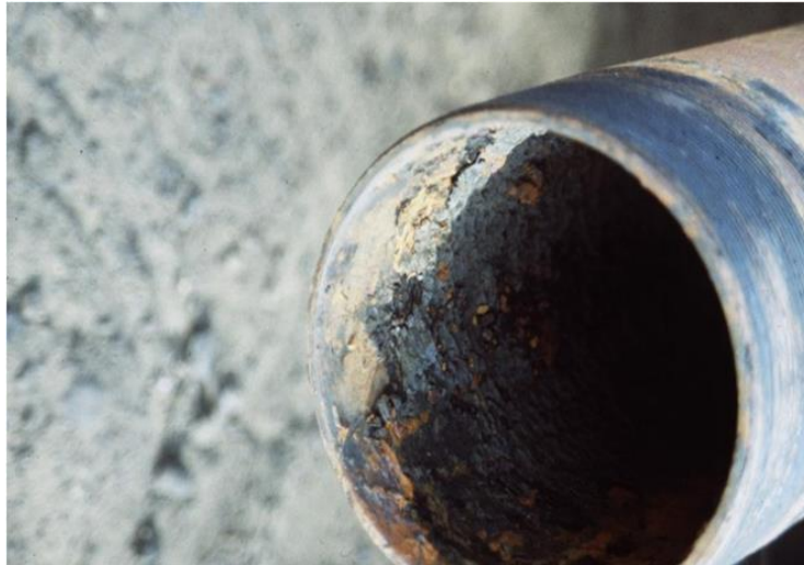
Fig. 2.4. A pipe affected by oxygen corrosion (taken from [46]).
