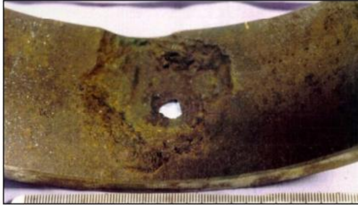
Fig. 2.9. A pit formed by sour corrosion (taken from [56]).
