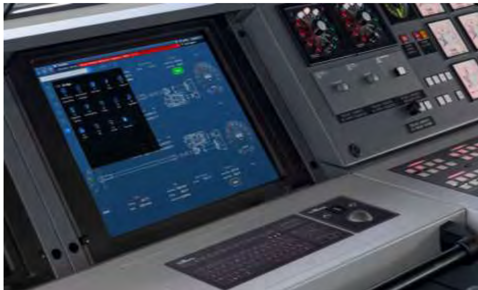
Picture 16 Alarm Monitoring and Control System (AMCS)
