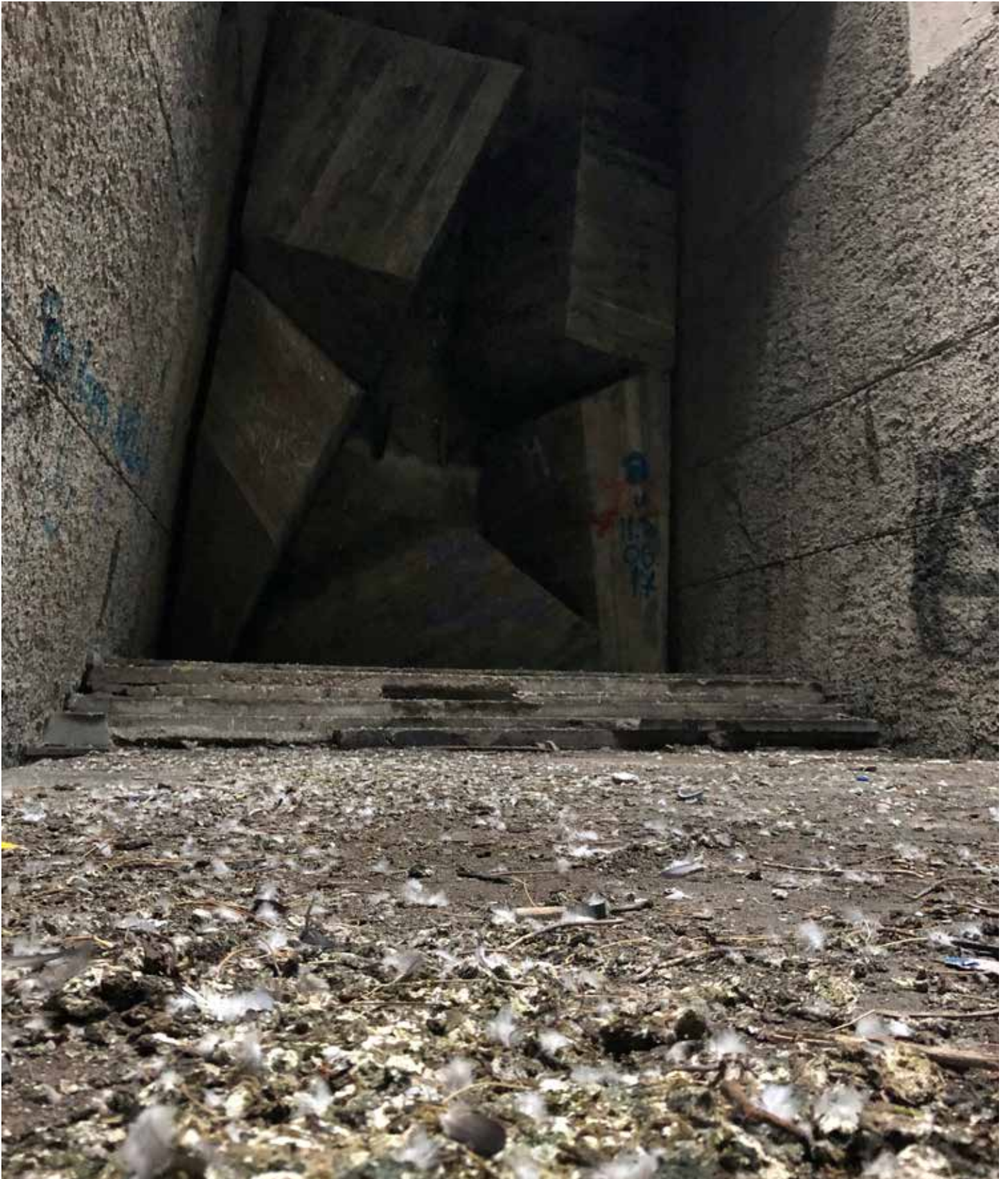
FIG 128. Pigeon feces covered ground underneath skylights
