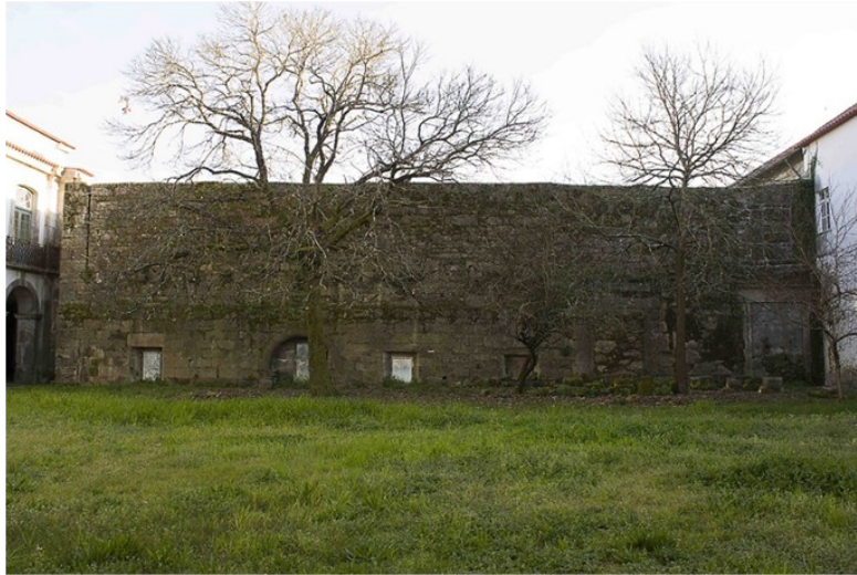
Fig. 8. The south wall of the south cloister, dating from the 16th century.
