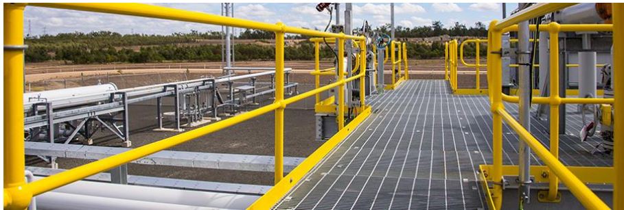
Figure 1. Steel grating platform (Access/Stainless Steel Grating - Flooring, Platforms, Access Systems, n.d.)
