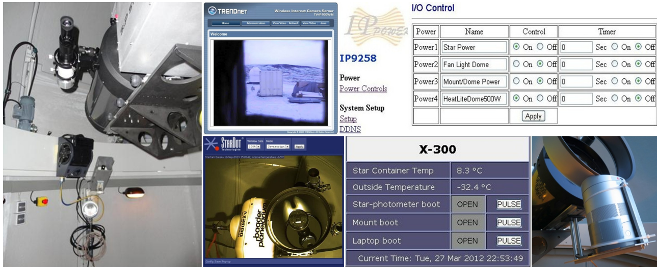
Figure 15: Remote maintenance kit (air blower, light projector, Vis/IR webcam); webcam views (from dome & OPAL); online panels for remote operations; testing Dyson blade-less fan.
