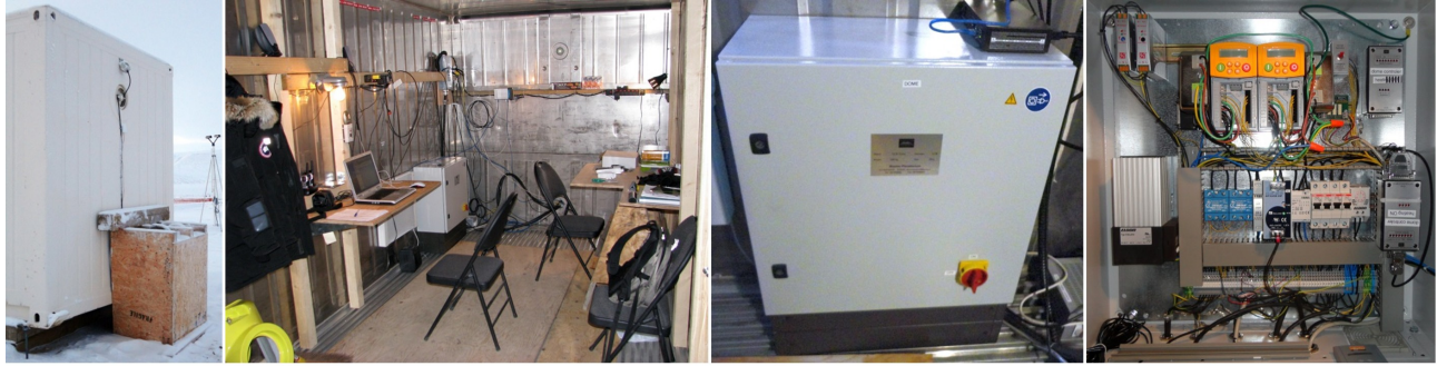
Figure 13: The sea-ship container transformed into a control room: cable protection and precipitation and temperature sensor; inside the control room; dome/mount high voltage unit; inside the unit.
