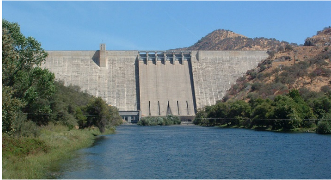
Fig. 1. A view of the CGD selected for modeling: the pine flat dam
