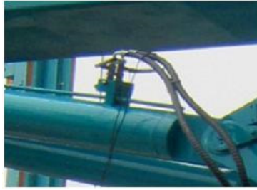
Fig. 12. Photograph of the pressure sensors installation location of the luffing cylinder
