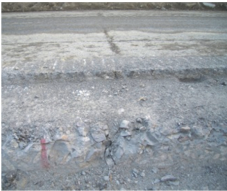
a) Transverse single crack
