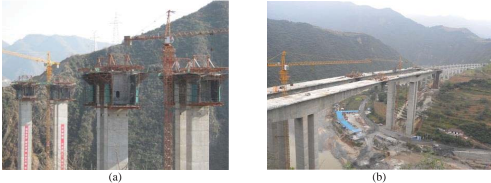
Fig. 5. Photos of a pre-stressed concrete Rigid Frame Bridge during different construction stage: (a) the zero block construction stage, (b) the closure up construction stage of the main span
