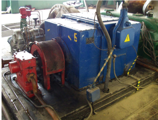
Fig. 1. General view of the electric motor-generator
