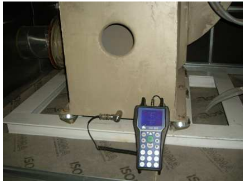
Fig. 6. The common view of the 1 st blower with stiffened foundation
