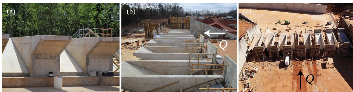
Figure 1. Overview of the new Piano Key weir (PK weir) under construction at West Fork of Eno Reservoir Dam (North Carolina, USA). (a) Looking upstream; (b) across weir towards right wingwall, and (c) looking downstream. Photos courtesy Schnabel Engineering.
