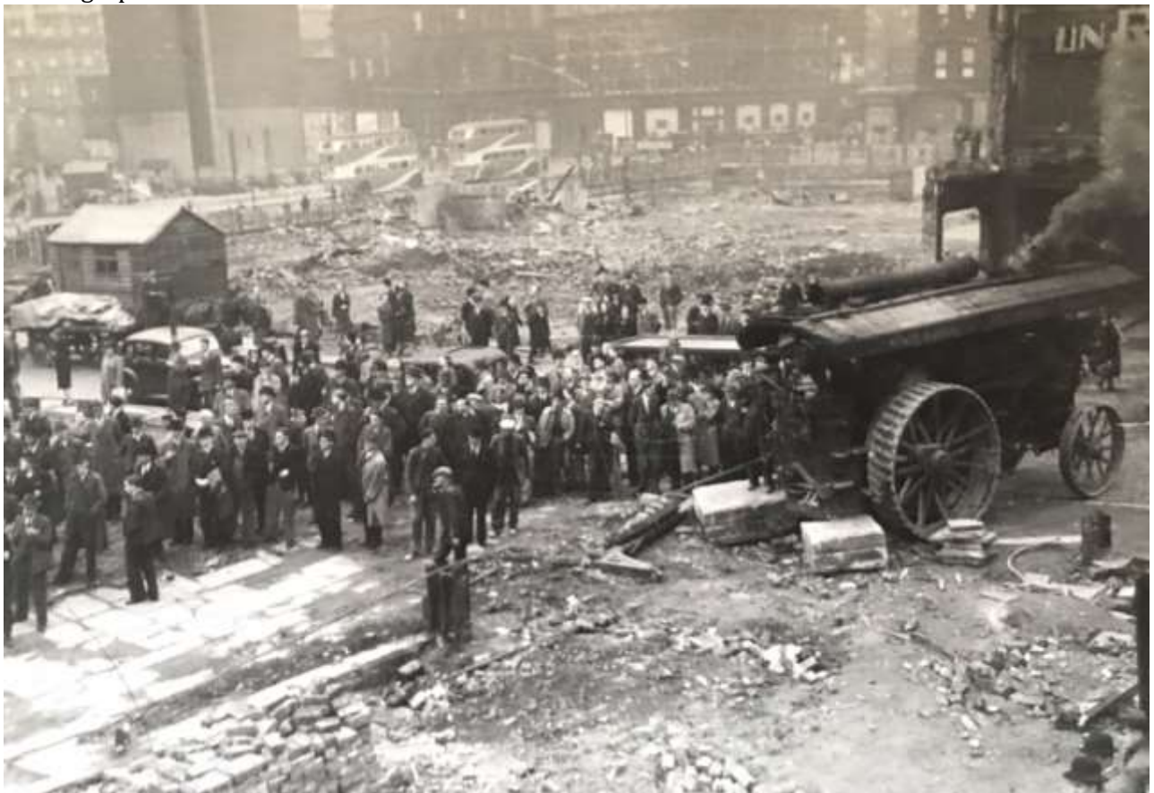
Appendix O – Fowler Showman’s Engine ‘King George VI’ photograph pulling down the bomb damaged Victoria Hotel in Manchester in 1941 whilst in the ownership of John P. Collins. Photograph from authors collection.
