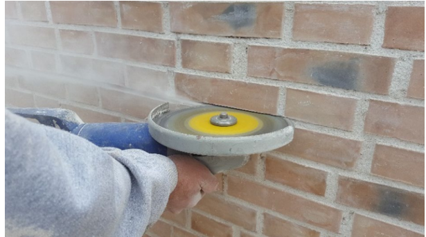
Fig. 8 The use of an electric disc cutter to make the slots for the steel cables
