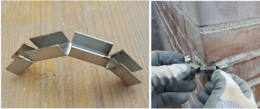
Fig. 10 Detail of a curved metal strip and its application: this was applied at wall edges (in the bed joint) and interposed between the masonry and the steel cable
