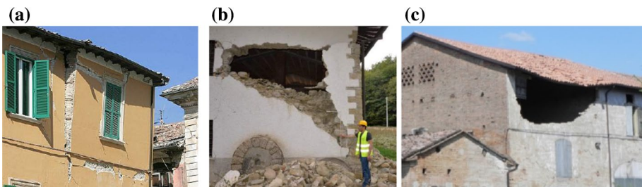
Fig. 14 Examples of out-of-plane mechanisms: a façade's out-of-plane rocking, b out-of-plane mechanism and shear/bending failure, c arch-mechanism
