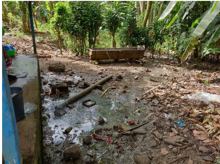
Figure 10: damaged washing station in Ilheu, rendering 2 sinks inoperable.
