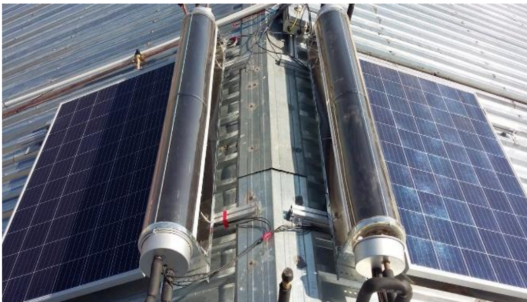
Figure 7: Rooftop installation at Jamataka primary school
