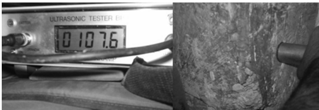
Figure 2: Process of Realization of the Ultrasonic Velocity Testing, Using a “Ultrasonic Tester”, in a Piece of Reinforced Concrete under Investigation
