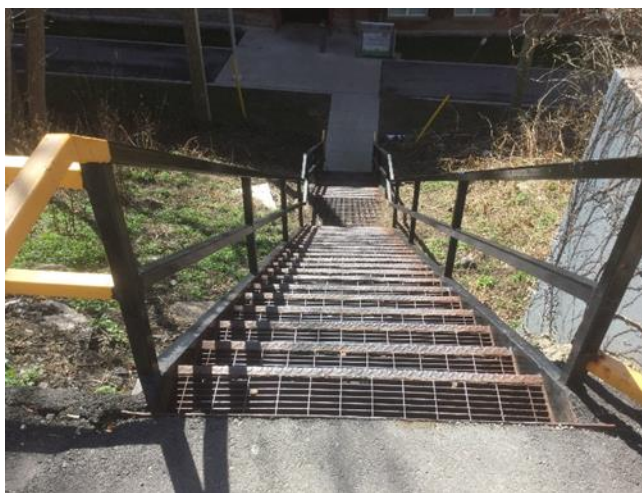
Figure 4.32. The steep metal staircase access to Marilyn I. Walker School of Fine and Performing Arts.
