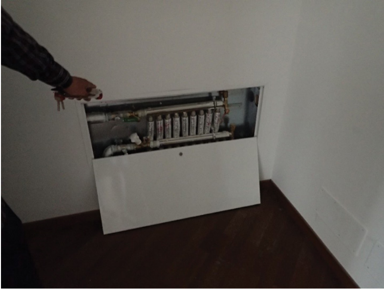
Figure 5.2 Tsogoo shows me the piping and valves behind the building's internal heating infrastructure as proof of their quality, revealing another European brand. Source: author
