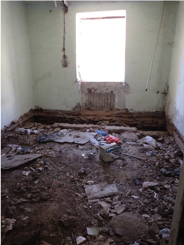
Figure 2.3 A room filled with waste has also had its heating pipes and radiator removed, and the glass taken from the window. Source: author
