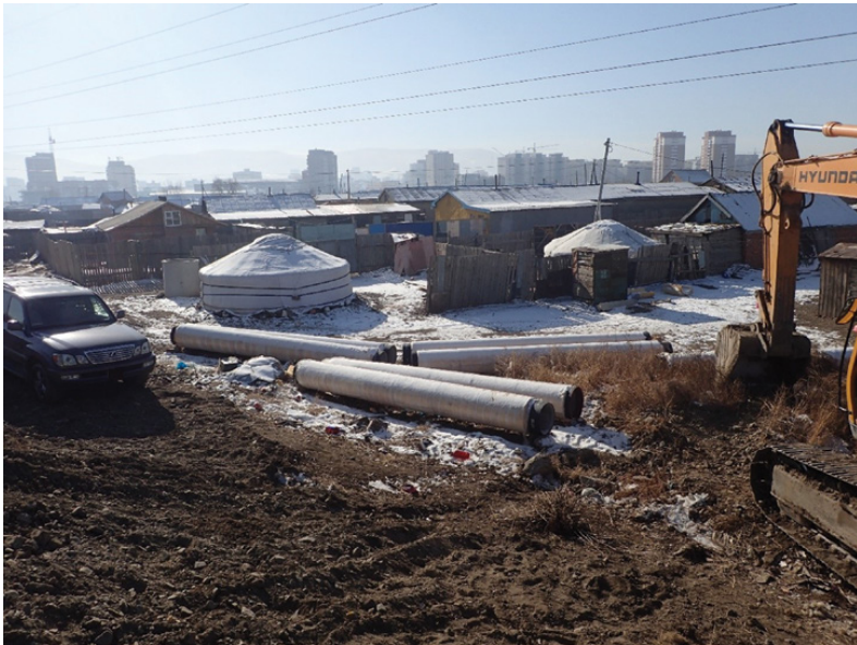
Figure 5.3 Promissory infrastructure: new sewerage pipes are laid north of the city, alongside expansive numbers of land plots not connected to core infrastructure. Source: author
