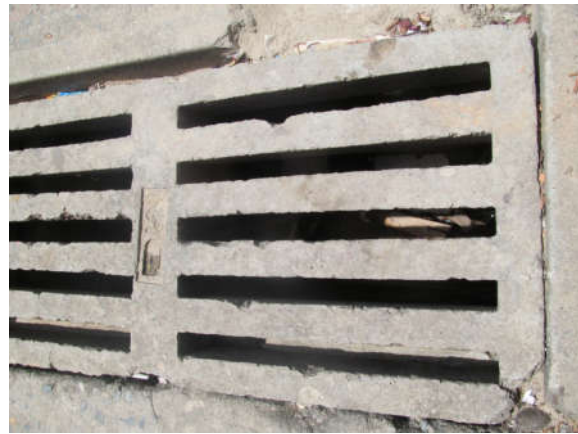
8-14 Debris hidden inside the drainage system
