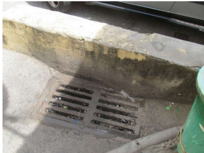
8-8 Drainage protected with screen
