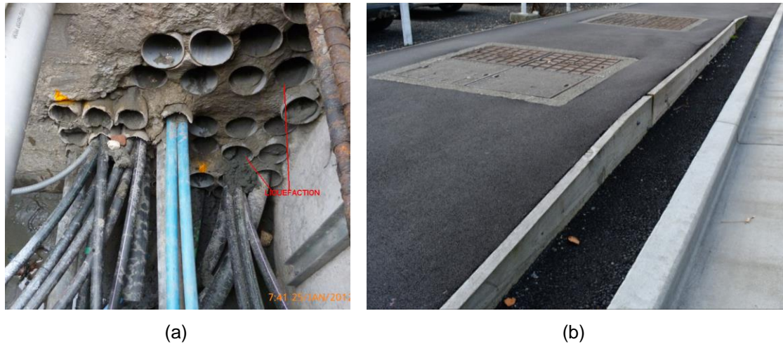
Figure 1. a) Liquefaction inside telecommunication ducts in a utility hole (Courtesy of Chorus Ltd) b) Uplifted utility hole in the CBD of Christchurch.
