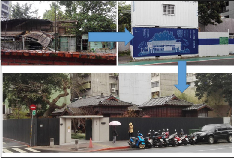
Figure 16.3 Traditional Japanese housing in Da'an district, around Jinhua Street, in different stages of rehabilitation. Photograph by Nicolas Zorzin, March–April 2016.
