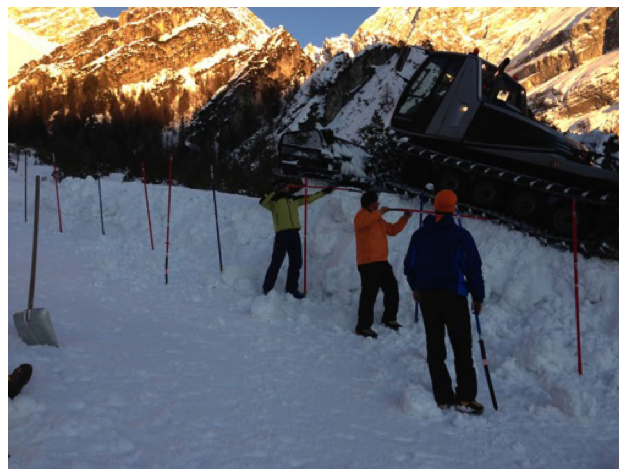
Fig. 1 In the process of constructing the constant EFH jump on the Antelao pitch of the San Vito ski resort
