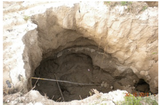
Figure 2. Signs of piping along the fissure. Soil erosion caused by water beneath the surface of the ground creating an underground tunnel.
