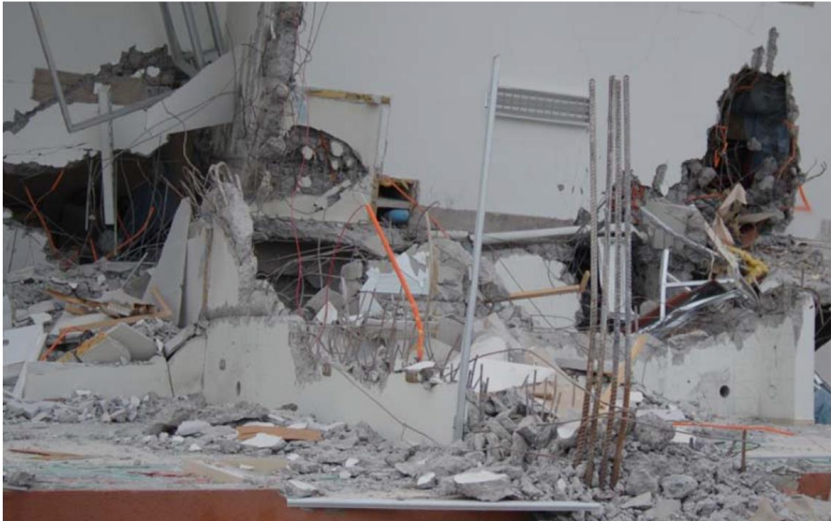
Figure 4 – Failure of lap splices reported by Song (2013).
