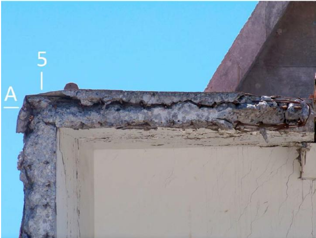
Figure 2 – Longitudinal splitting observed in Concepcion, Chile, Alto Rio Building, 2010 (Song, 2013).
