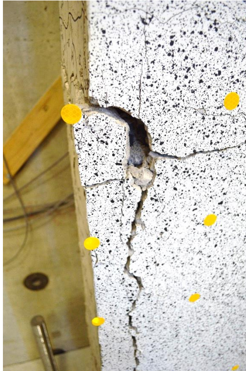
f. W80C Splice Failure (South East Edge)
