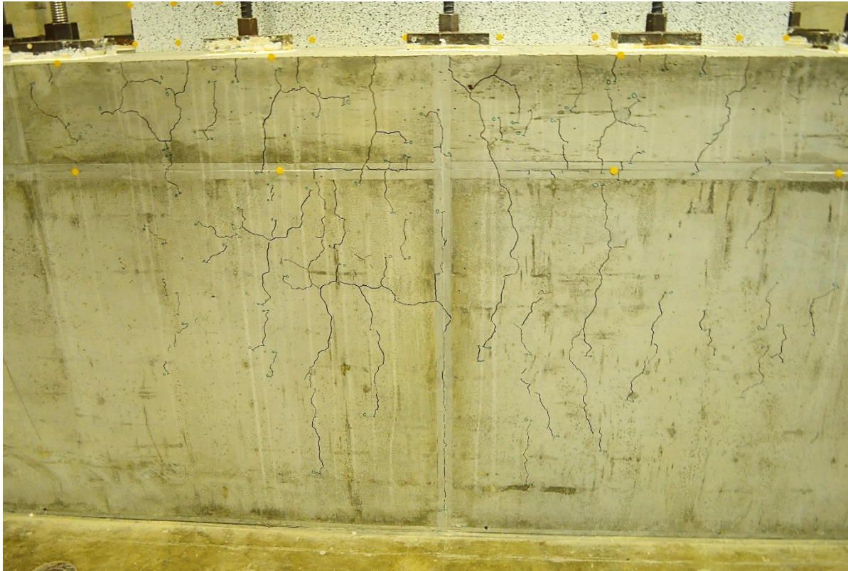
Figure 49 – Shrinkage Cracks observed and marked on the foundation of Test Wall W80C.
