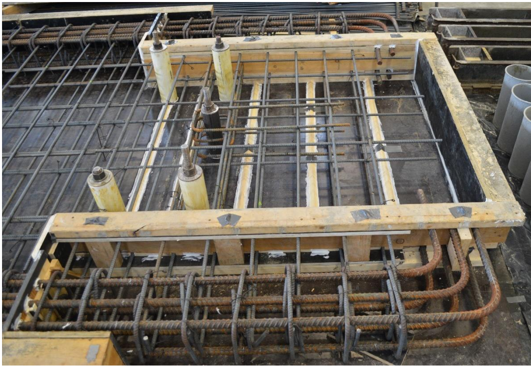
Figure 43 – Photographs of formwork built around spliced reinforcement near base of test wall.
