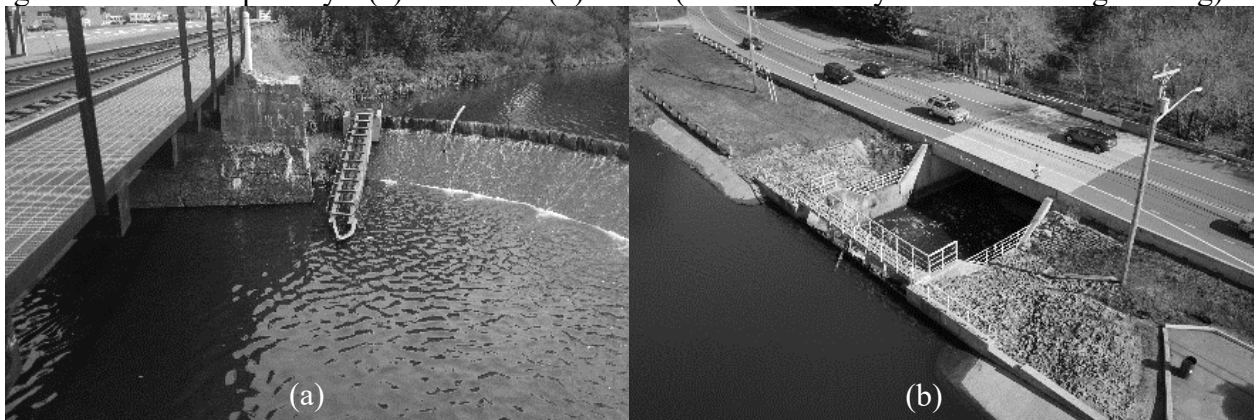
Fig. 1 – Modelled Spillways: (a) Site 1 and (b) Site 2 (Photos courtesy of Schnabel Engineering)
