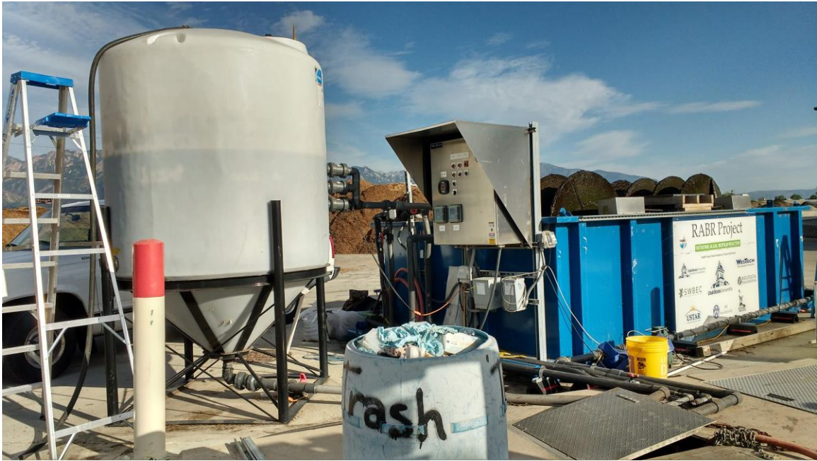
Figure 2. This is the west-facing side of the CVWRF RABR. AD filtrate flows into the white settling tank on the left side then flows into the blue RABR tank.
