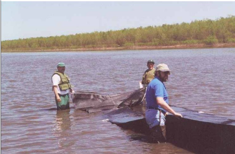
Figure 10. Small geotextile tubes were placed in Upper Peoria Lake near Chillicothe in the Spring of 2001. When filled with sediment the tubes formed a small trapezoidal island. The tubes are intended perform like a berm, hold the sediment in place, and prevent it from being eroded by wave action.
