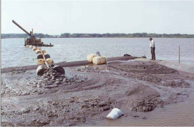
Figure 11. The Dry Dredge shown here lifts sediment from the lake bottom and uses a displacement pump to move it without adding water. The pump filled the geotubes with sediment and then pumped sediment with the consistency of toothpaste behind the tubes to form a small island. The island was filled on May 2.
