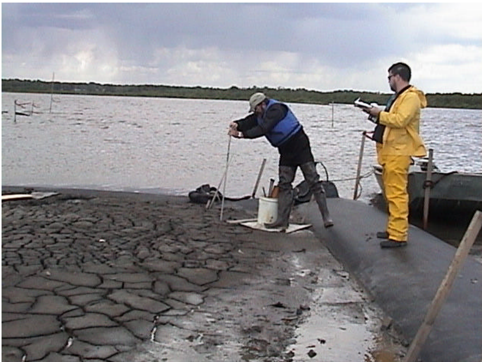
Figure 8. Engineers taking measurements at a demonstration island three weeks after it was constructed using soft sediment in Upper Peoria Lake. To the right is a small geotextile tube used to protect the island from waves and hold the sediment in place while it consolidates. The sediment was excavated and pumped with the DRY DREdge™ at about 40 cubic yards per hour.
