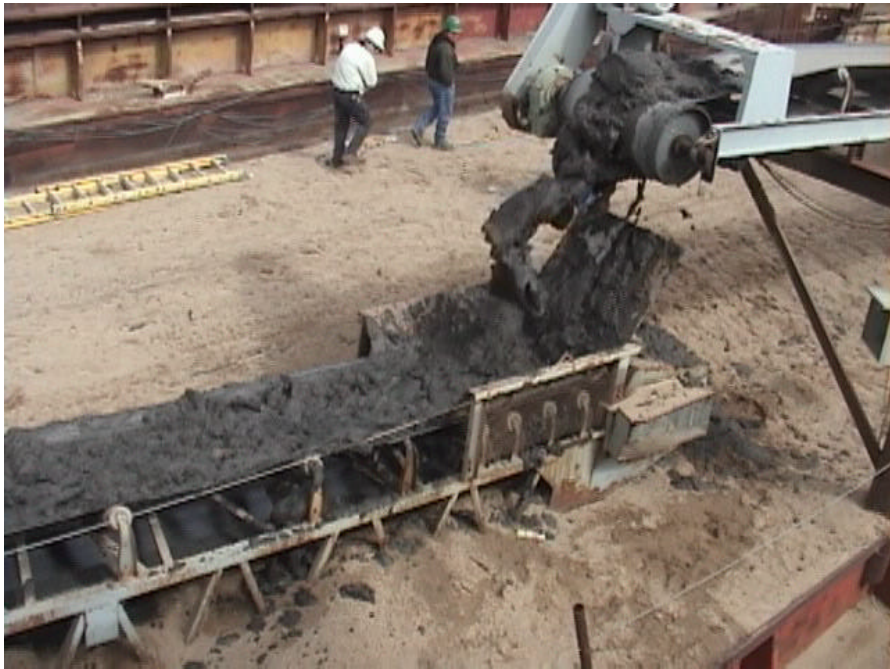
Figure 10. Peoria Lake sediment passing through a transfer point at a sand pit. The conveyor system was designed for sand and no modifications were made for the sediment. The material did not liquefy or build up excessively on the belts or chutes. Belt scrapers and transfer points could be specifically designed for sediment.
