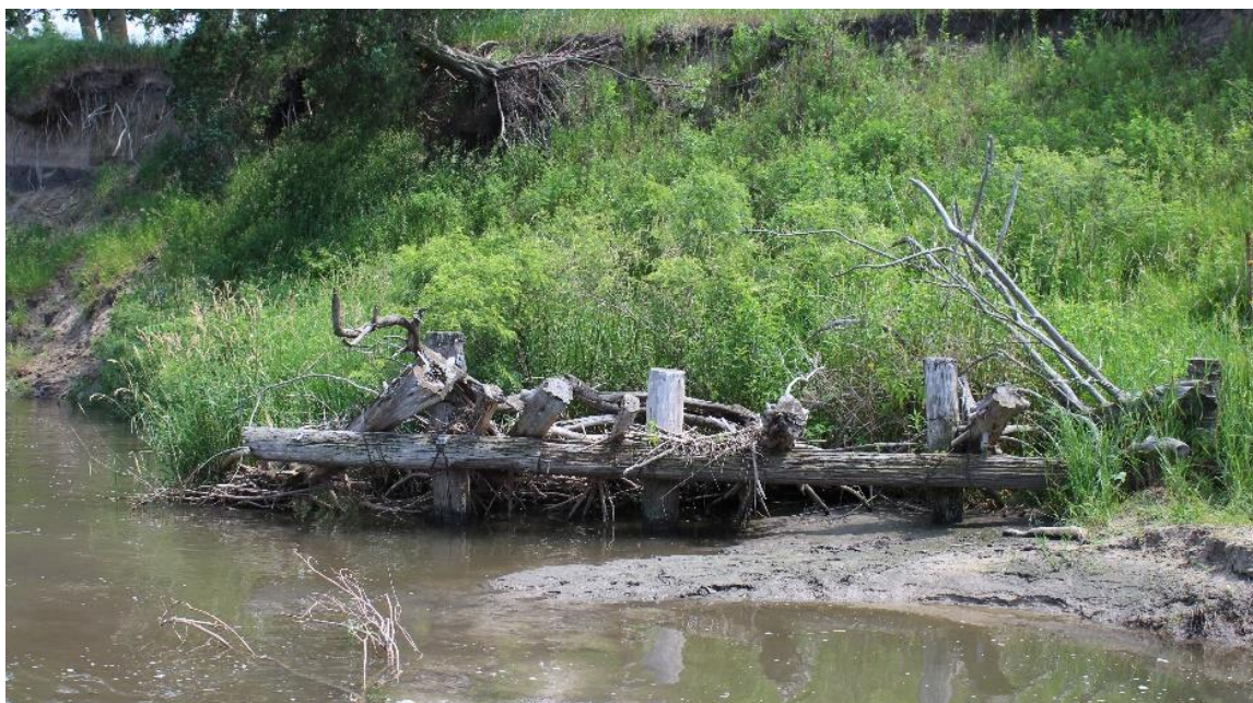
Figure 2. An image of the wooden jetty structures used on Cedar River as part of the Cedar River Stabilization Project
