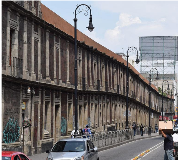
Figure 2.3 - Visible differential settlement in a building constructed on lake bed in Mexico City (Nikolaou et al., 2018).
