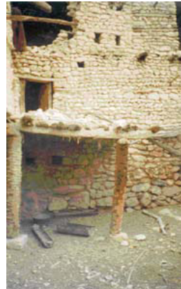
Figure 6: A covered area in the courtyard provides a protected against heat and glare space.
