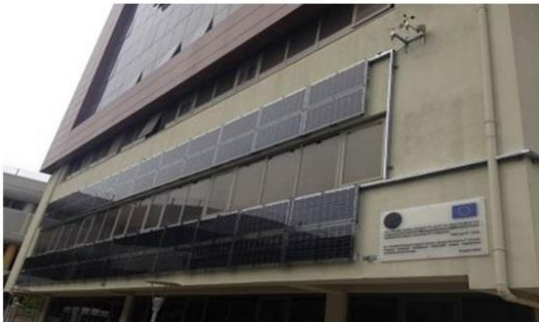
Figure 2. A picture of the BIPV system (Araz et al., 2017).
